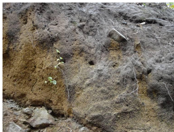
Fig. 5 Piping holes in the topsoil layer located on the lower part of slope
