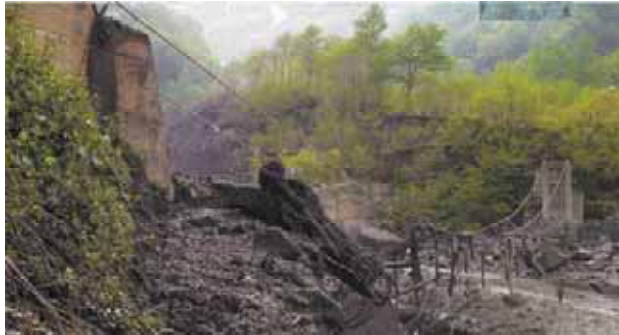
Fig. 6 The suspension bridge that was completely destroyed by the May 2004 debris flow in the Bettou-dani (Photo courtesy of the Kanazawa Office of Rivers and National Highways, MLIT)
